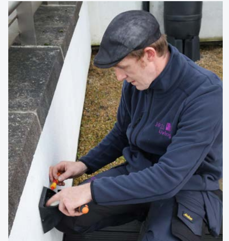
I-RES Maintenance Technician, Karl Seery upgrading the Common Area LED lighting at Kings Court, Dublin 7
