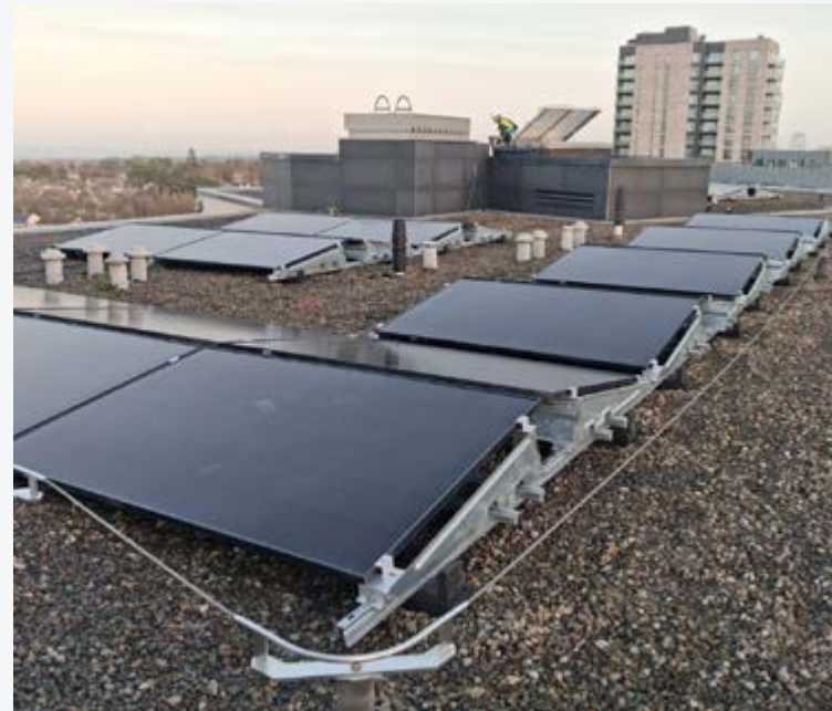
Solar Panels at Rockbrook, Dublin 18
