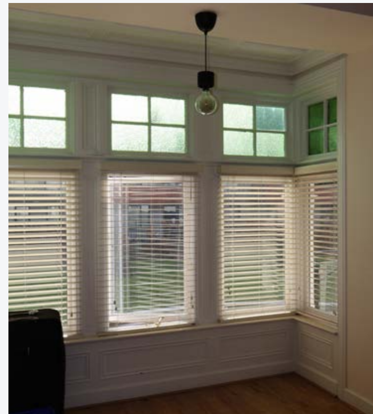
2 bed, Bessboro, Dublin 6W with original single glazed timber fit windows, before upgrade
