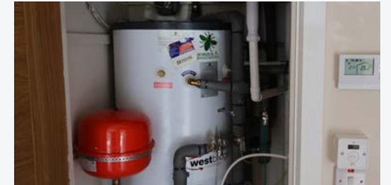
Upgraded energy-efficient Viessmann heat pump system
