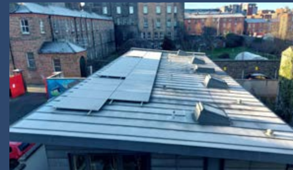
Solar Panels at Xavier Court, Dublin 1
